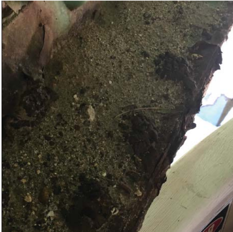
Photo #39: Remnants of rivet heads along the top of the bottom flange of the bottom chord of the sidewalk truss (western) in span 3 (8/2/16)
