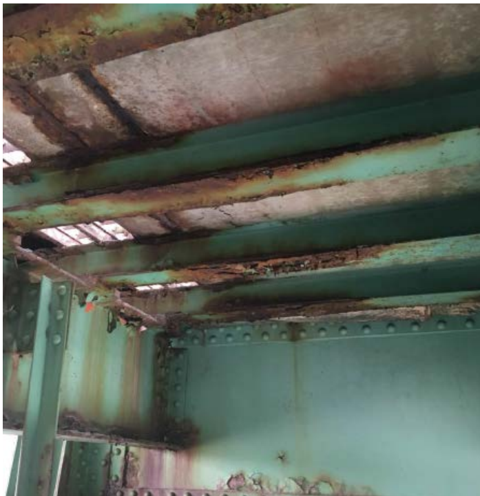
Photo #42: Typical view of cross beams (needle beams) in the exterior bay between S3 & S4, S7 & S8 similar (8/1/16)
