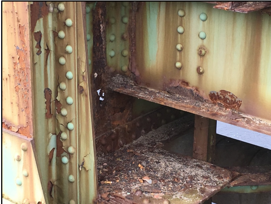
Photo A1 – Floorbeam 7, Roadway Truss @ Stringer 8 (Exterior)
