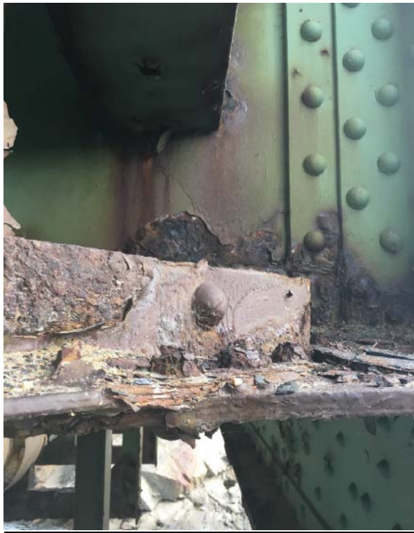
Photo #54: Corroded lateral bracing end at its connection to the horizontal plate at FB8 span 2 (8/2/16)
