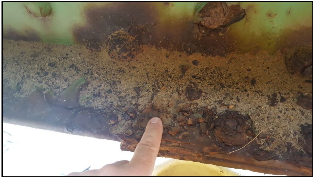
Photo A5 – Floorbeam 5 coverplate has enough deterioration issues to expect a repair within 5 years.
