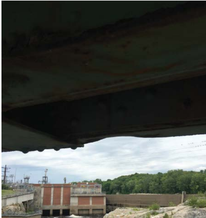
Photo #41: “Dent” to the exterior member making up the bottom chord on the sidewalk (western) truss at the same location of the previous photo (8/1/16)
