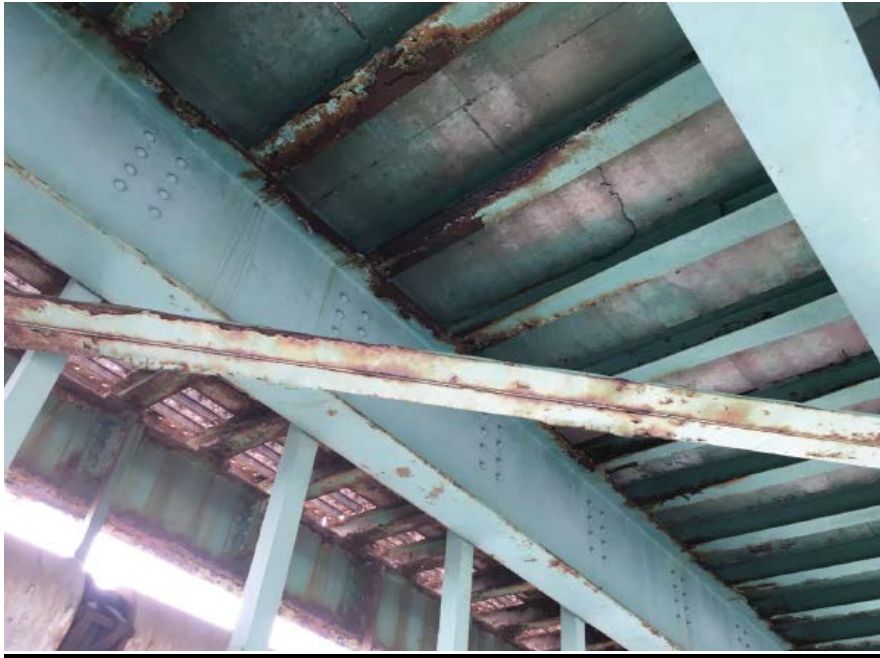
Photo #43: Typical view of cross beams (needle beams) in the first interior bays from S4 through S7 (8/1/16)
