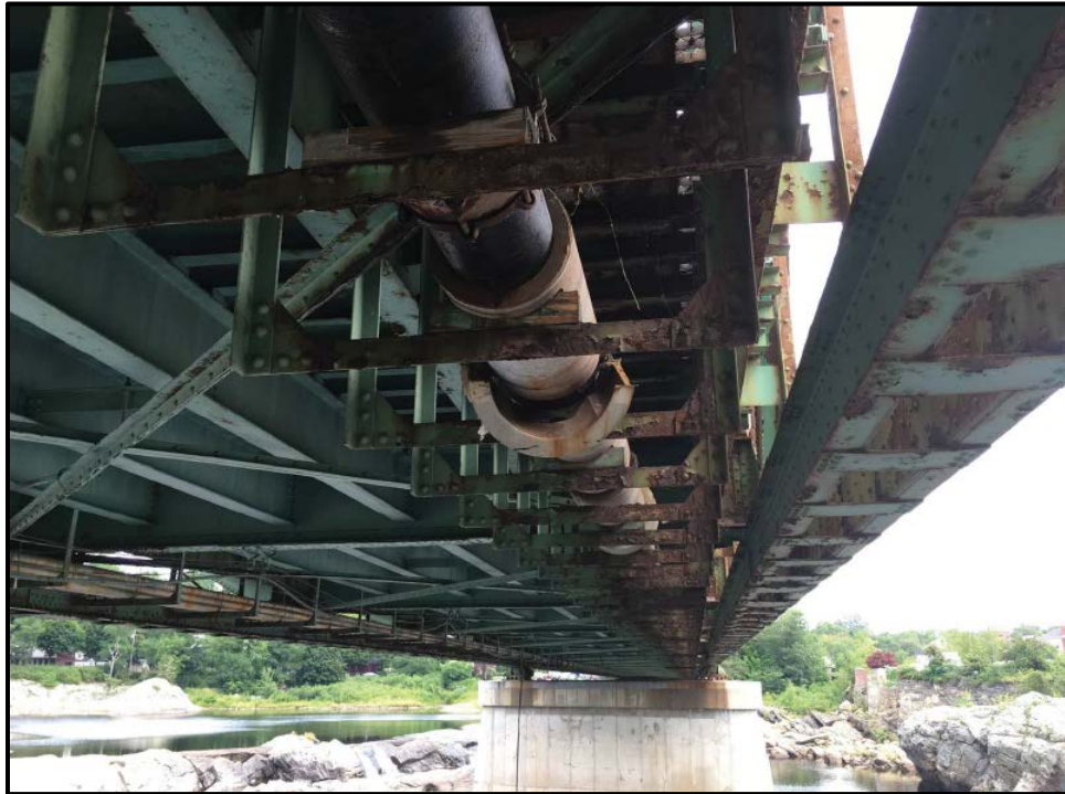
Photo A23 – View of steel insulated utility pipe extending across the bridge on the Roadside Truss side.
