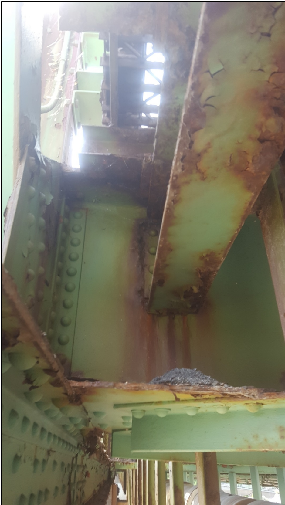
Photo A16 – Stringer 8 connection to Floorbeam 2 will likely need repair within 5 years.
