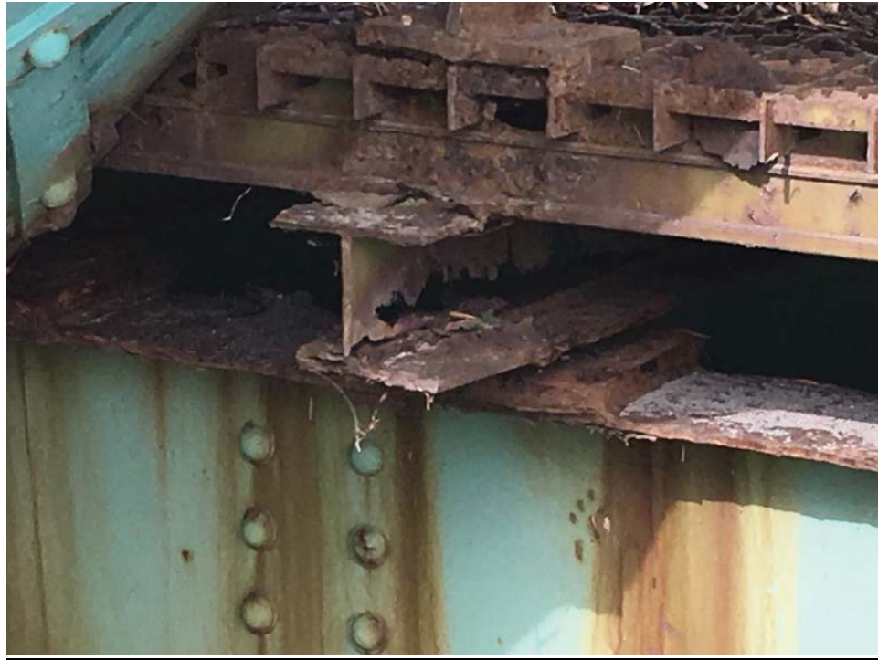
Photo #45: Severe corrosion to a cross beam (needle beam) near FB 1 in span 1 of non-sidewalk (eastern) truss (8/1/16)
