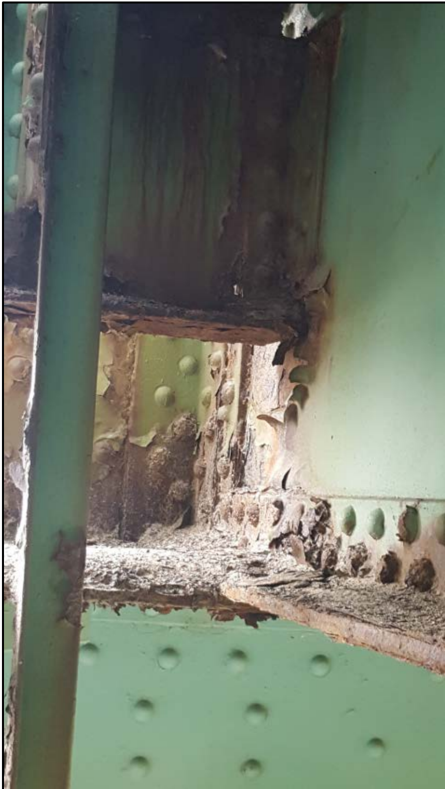
Photo A12 – Stringer 8, Roadway Truss @ Floorbeam 2 has section loss revealing a web hole.
