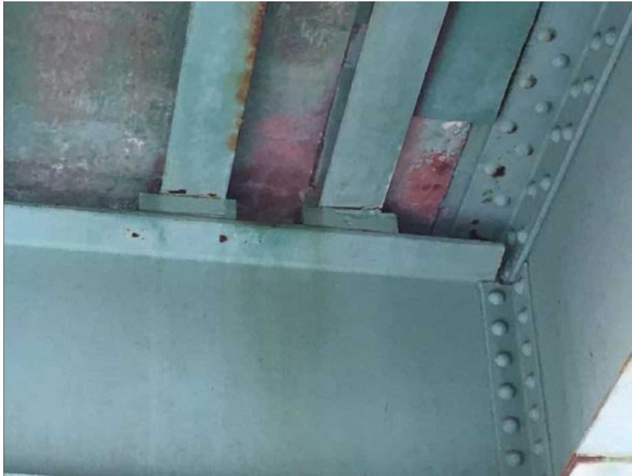
Photo #47: Failed weld between needle beam and an interior stringer in span 1 (8/1/16)
