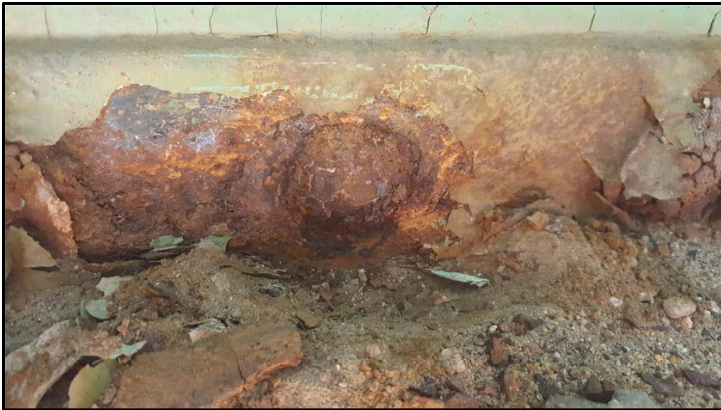
Photo A10 – This is the same rivet as above after briefly pounding loose corrosion away. The rivet head size is significantly smaller than the diameter and height of a new rivet head.
