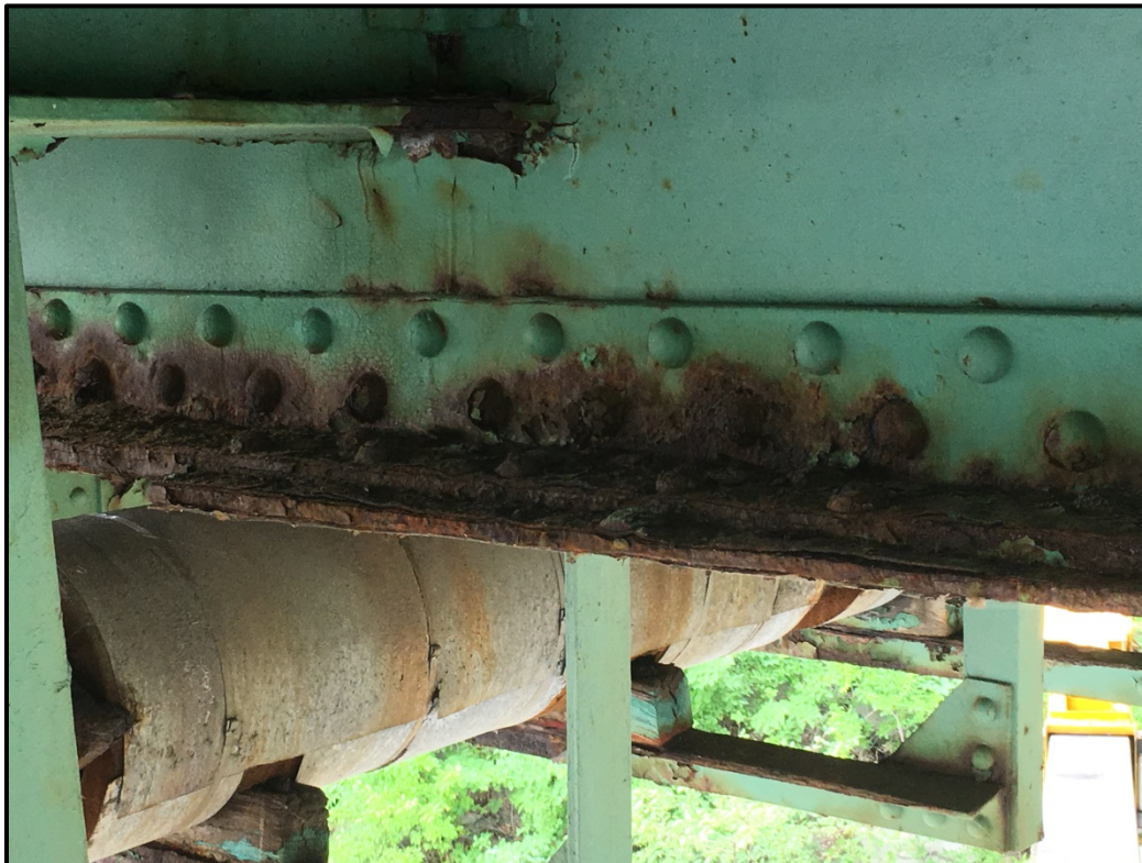
Photo A4 – Floorbeam 2 coverplate particularly between Stringer 7 & 6 is an area of concern which will be closely monitored.
