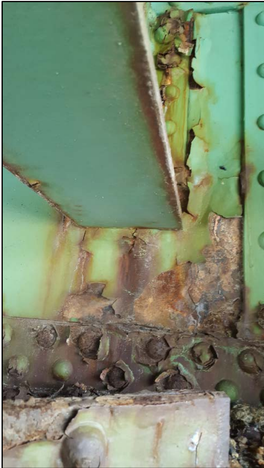
Photo A13 – Looking at the condition of north end of Stringer 8 attached to Floorbeam 3.
