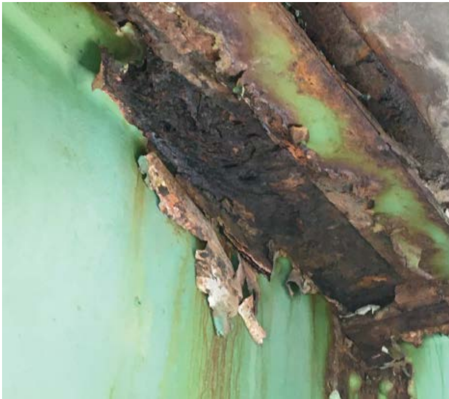
Photo # 22: Top flange corrosion & section loss of FB 5 in span 3 (8/2/16)
