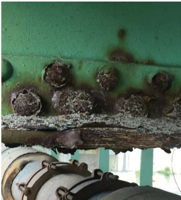
Photo # 20: Advanced deterioration of rivets near midspan of FB7 in span 2 (8/2/16)
