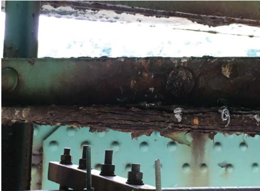
Photo #55: Pack rust and section loss to the lateral bracing near FB6 in span 1 (8/1/16)
