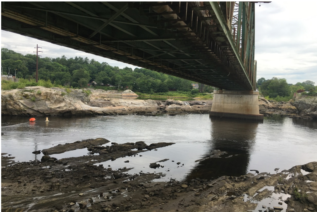
Photo #2: General view of the underside of the non-sidewalk side of the bridge (eastern side, Span 1 looking north) (8/1/16)
