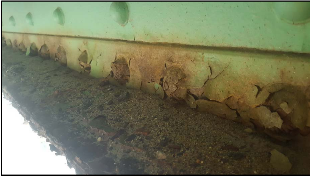
Photo A8 - View of the inside of Sidewalk Truss's lower angle depicts continuous corroding rivet heads and sand, salts and debris occupying the angle flange.
