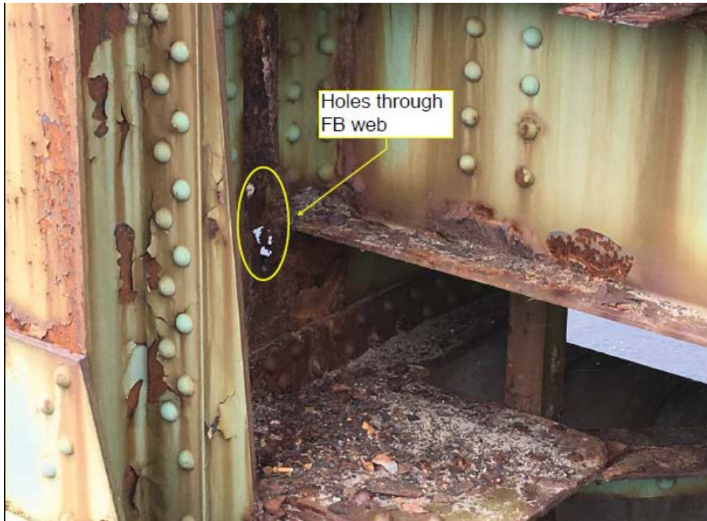
Photo # 15: General view of corrosion and holes through the web of non-sidewalk (eastern) end of FB7 in span 1 (8/1/16)
