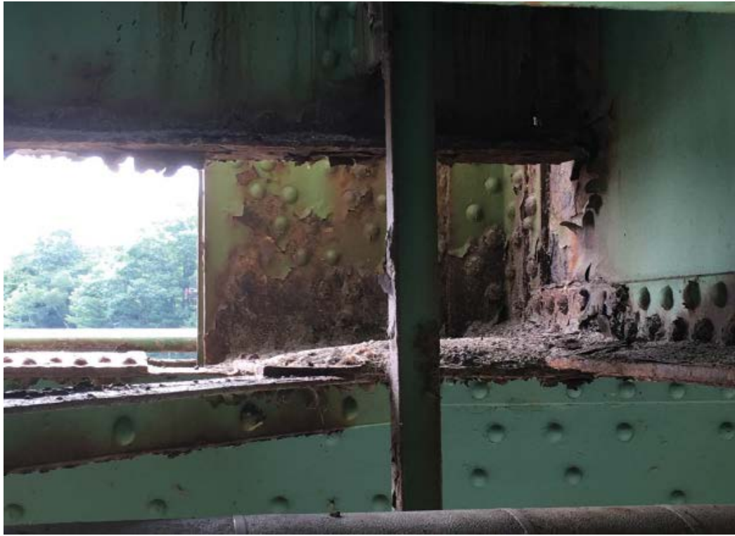
Photo # 11: General view of typical paint loss & debris collection at floor beam ends (8/1/16)
