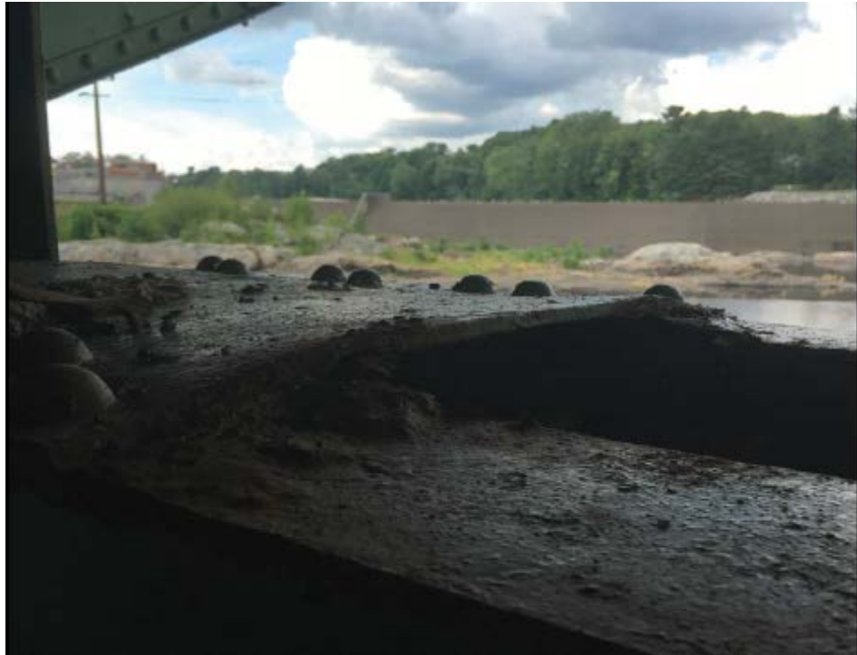
Photo #33: “Bowing” of lattice plates on the top of the bottom chords of the sidewalk truss in span 3 (8//16)
