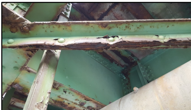
Photo A26 – In general, a good amount of deterioration exists in the lateral bracing system.
