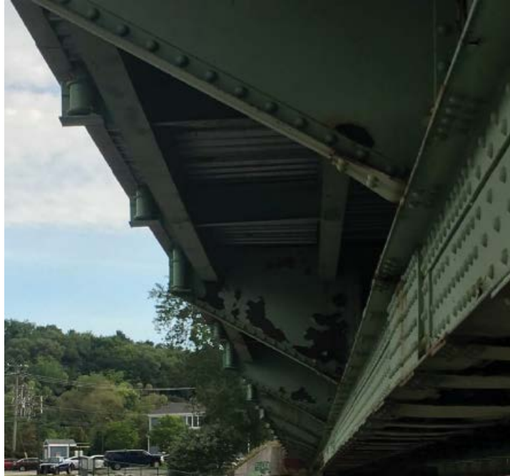
Photo #23: Typical view of the sidewalk stringers (S1 & S2) on the upstream side of the bridge (western side, looking north) (8/1/16)
