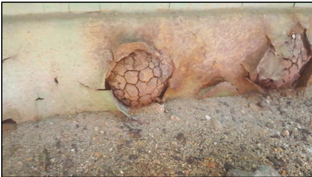
Photo A9 - Typical rivet head condition along Sidewalk Truss Lower Chord of Span 3 for at least 100 ' length of angle to plate connection.
