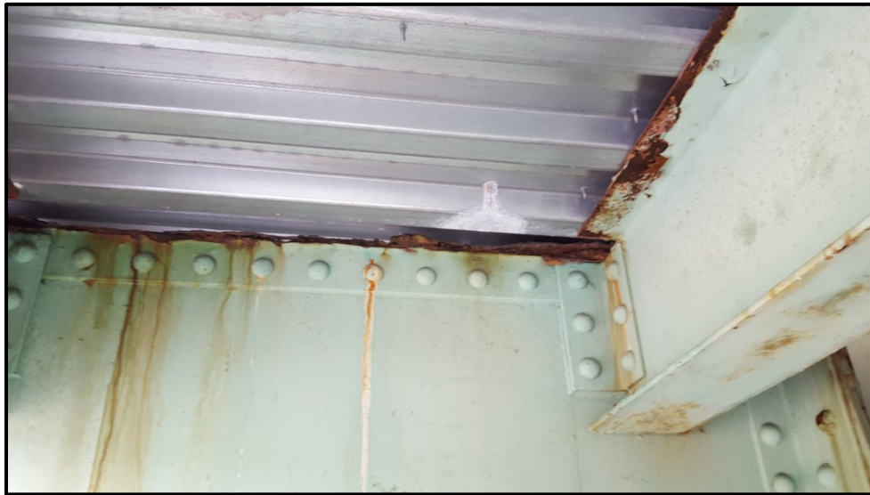
Photo A25 – View of the top half of cantilevered brackets that support the sidewalk.
