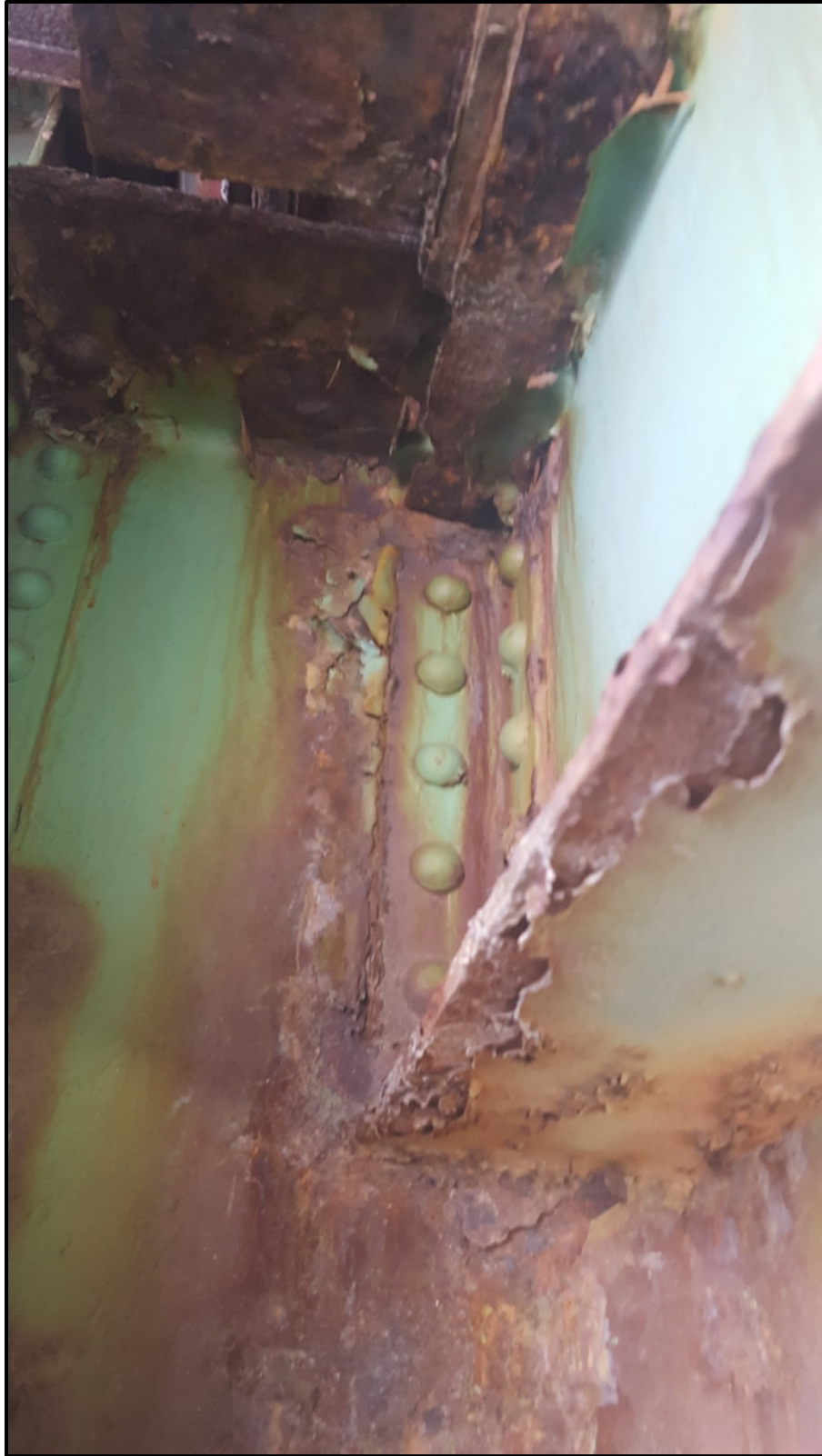
Photo A19 – Stringer 8 connection to Floorbeam 6 will likely require repairs within 5 years.
