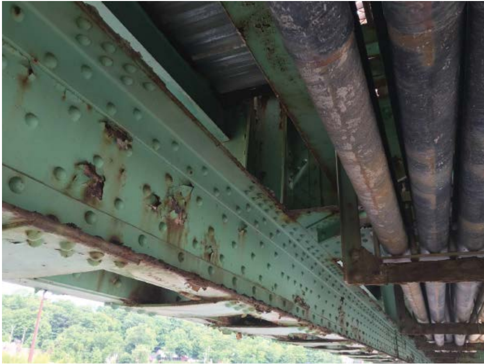
Photo # 9: General view of paint loss and corrosion to bays below the open grid decking in the travel way shoulders on the sidewalk side (western) of the bridge (8/1/16)
