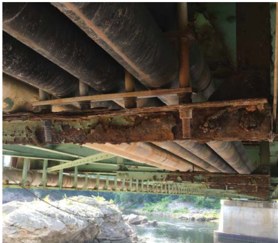
Photo #6: General view utility conduit supported by a hanger system attached to the stringers (western side of structure looking south) (8/1/16)
