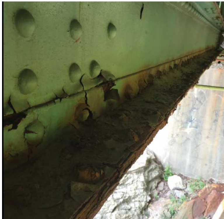
Photo #36: Corrosion to the bottom flange of the bottom chord of the sidewalk side truss in span 3 (western side of the bridge looking north) (8/2/16)
