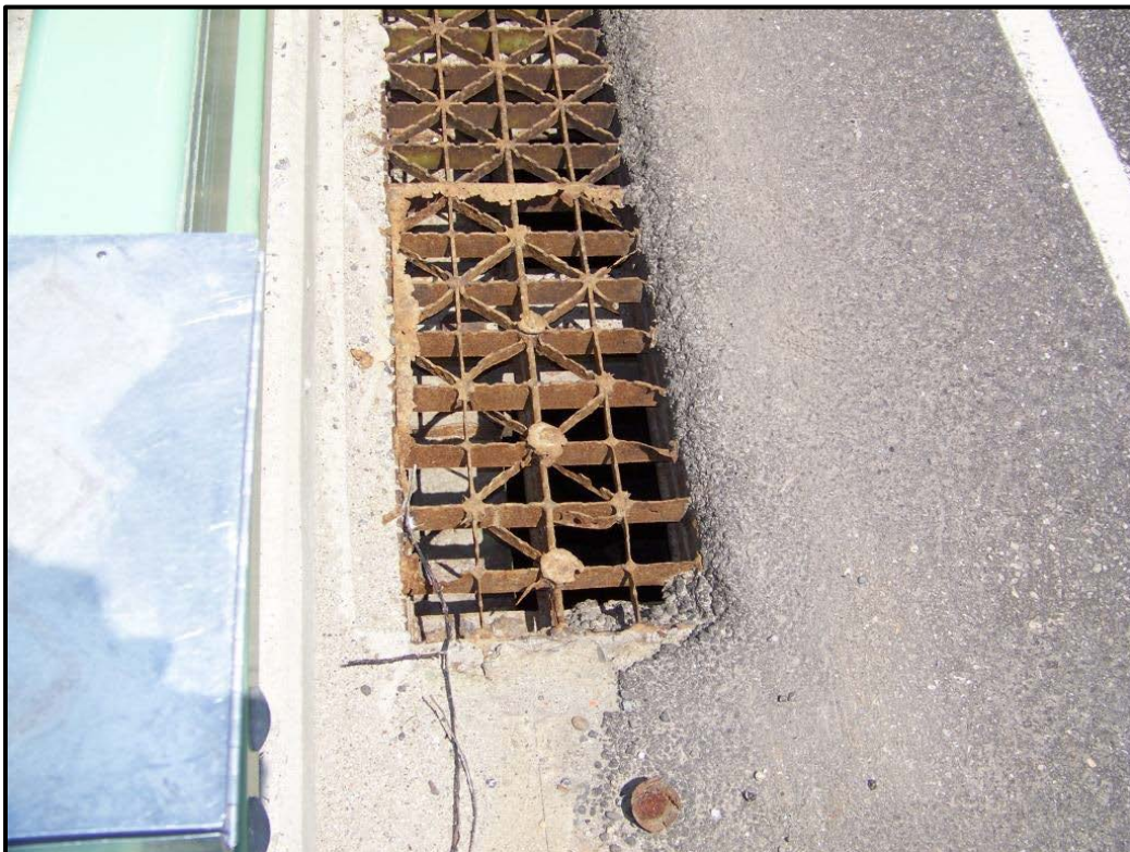
Photo A22 – An open grid approximately 1 foot wide runs parallel to Stringers.
