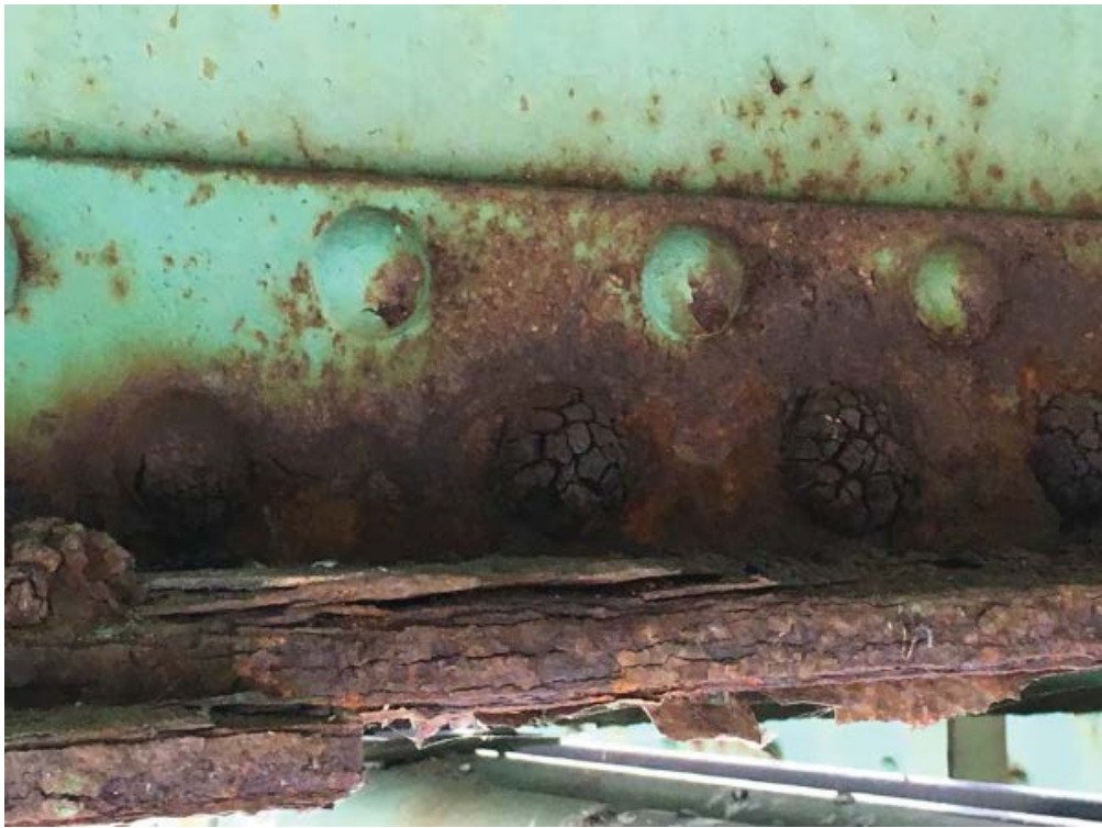
Photo # 19: Severe corrosion to the rivets as well as corrosion & pack rust between the bottom flange of the floor beam and the cover plate near midspan of FB5 in span 2 (span 2 FB4, FB6 & FB7 similar) (8/2/16)
