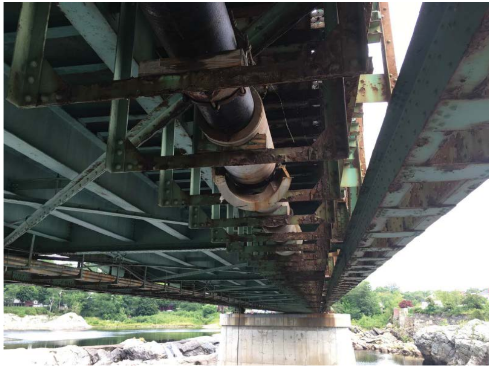
Photo #7: General view of utility pipe supported by a hanger system attached to the stringers (eastern side of structure looking north) (8/1/16)
