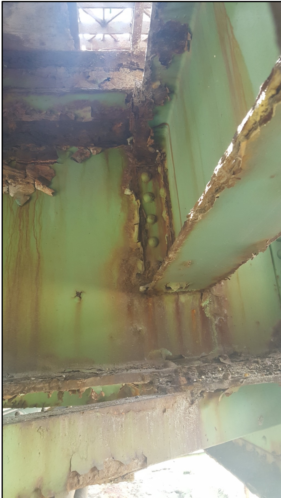
Photo A18 - Stringer 8 connection to Floorbeam 6. Stringer 3 connection similar condition.
