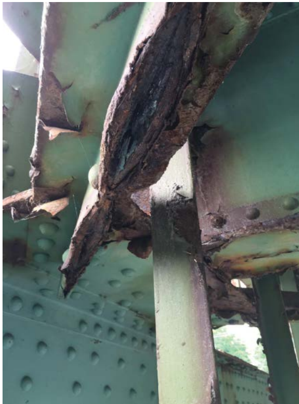
Photo #51: Severely corroded lateral bracing member, view from the bottom of the double angle connections in Spans 1 & 2 (8/1/12)
