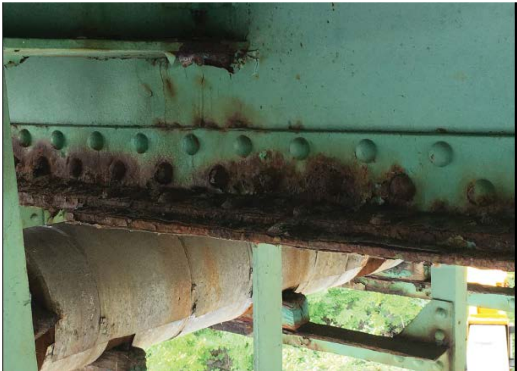
Photo # 18: Severe corrosion & pack rust between the bottom flange of the floor beam and the cover plate near midspan of FB5 in span 2, (span 2 FB4, FB6 & FB7 similar) (8/2/16)
