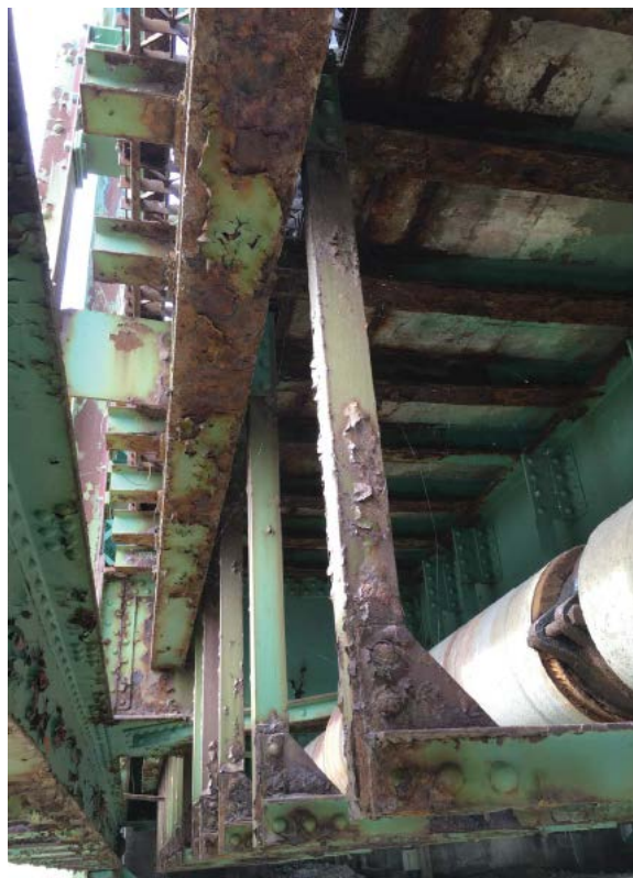
Photo # 8: General view of paint loss and corrosion to bays below the open grid decking in the travel way shoulders on the non-sidewalk side (eastern) of the bridge (8/1/16)
