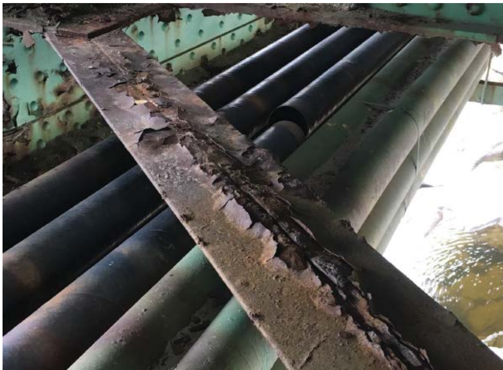
Photo #50: Severely corroded lateral bracing member view from top of double angle in spans 1 & 2 (8/1/12)
