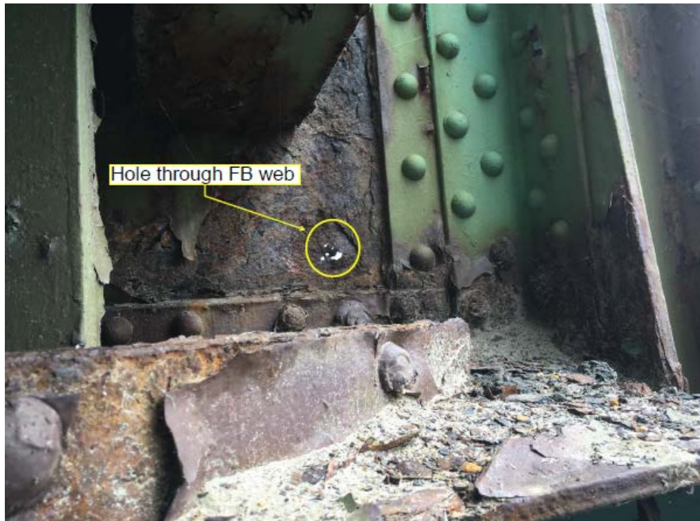
Photo # 14: General view of corrosion and hole through the web of the non-sidewalk (eastern) end of FB5 in span 1 (8/1/16)
