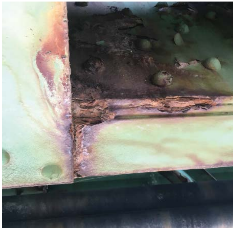
Photo #34: Pack rust between lattice plate and bottom angle on the the bottom chord of the sidewalk truss in span 3 (8//16)
