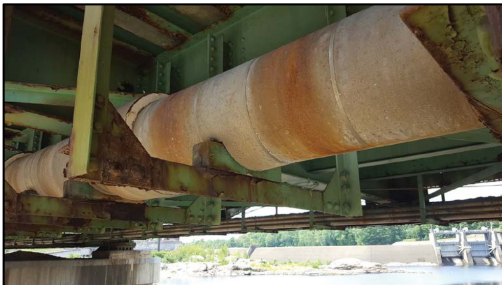
Photo A24 – The Utility Brackets are in poor condition with extensive active corrosion.
