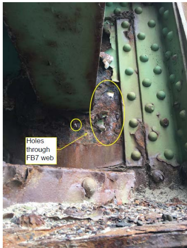
Photo # 16: Closer view of holes through the web of FB7 (8/1/16)
