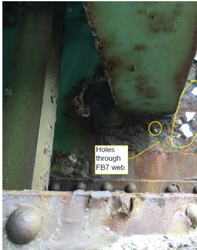
Photo # 17: Closer view of holes through the web of FB7 (8/1/16)
